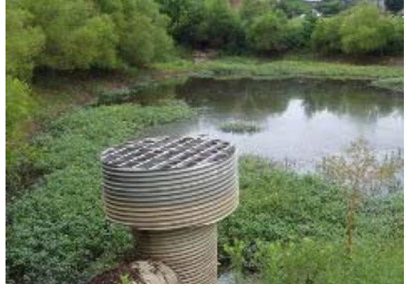
Non-compliant pond with failed riser.
