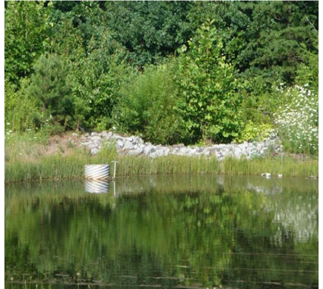
Non-compliant pond due to vegetation growing in emergency spillway.
